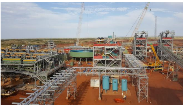
Photo 5 View from HPGR feed bin facing the DMS
