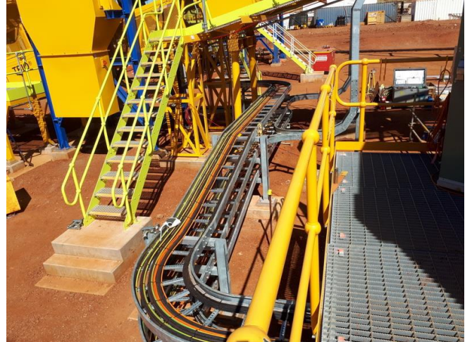
Photo 5 Cable Installed in the Crusher
