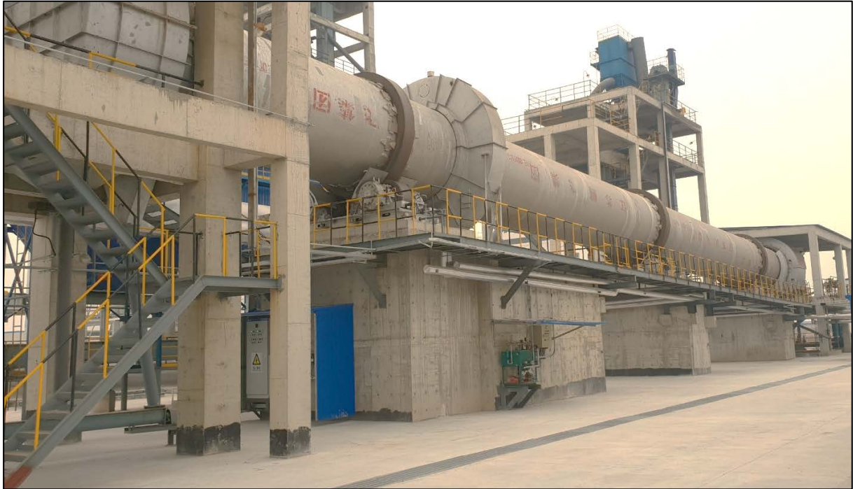
Rotary Kiln at the Tianyuan Plant
