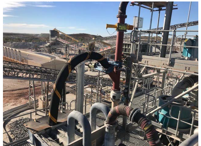
Photo 3. New By-Pass System
